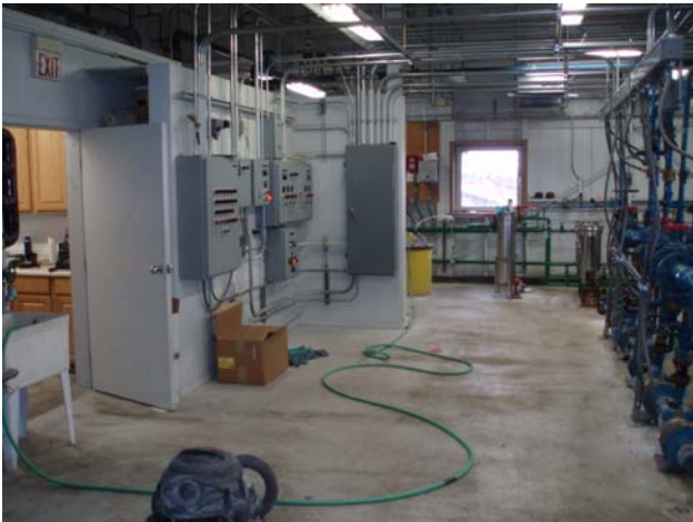
S13 Building Mid-Line and Electrical Panels
