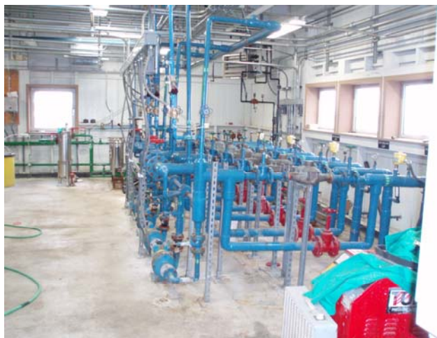
S07 Loop Circulator Piping Manifold
