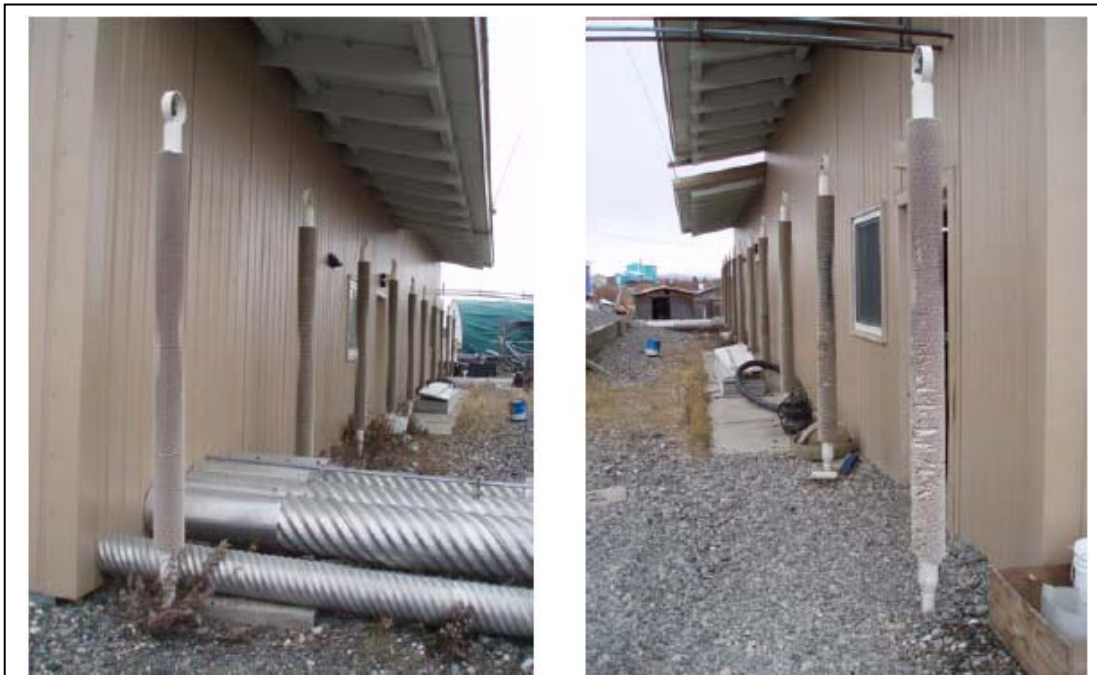
Figure 4. Thermosyphons along West Wall (Looking South & North)
