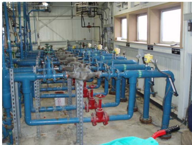
S08 Loop Circulator Piping Manifold
