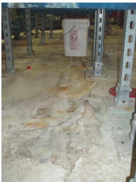
S11 Floor Cracks Along Settlement Line Below Water Circulation Manifolds
