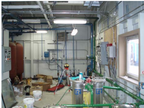
S10 Cartridge Filters and Pressure Pump
