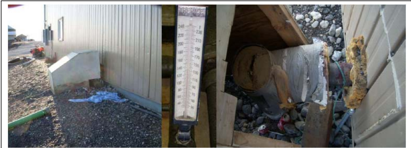
Figure 5. Waste Heat Circulation Line at Water Treatment Plant
