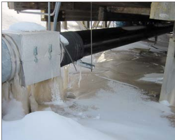
A leaking junction between the main water line and a house. Jake Bell, 2014.
