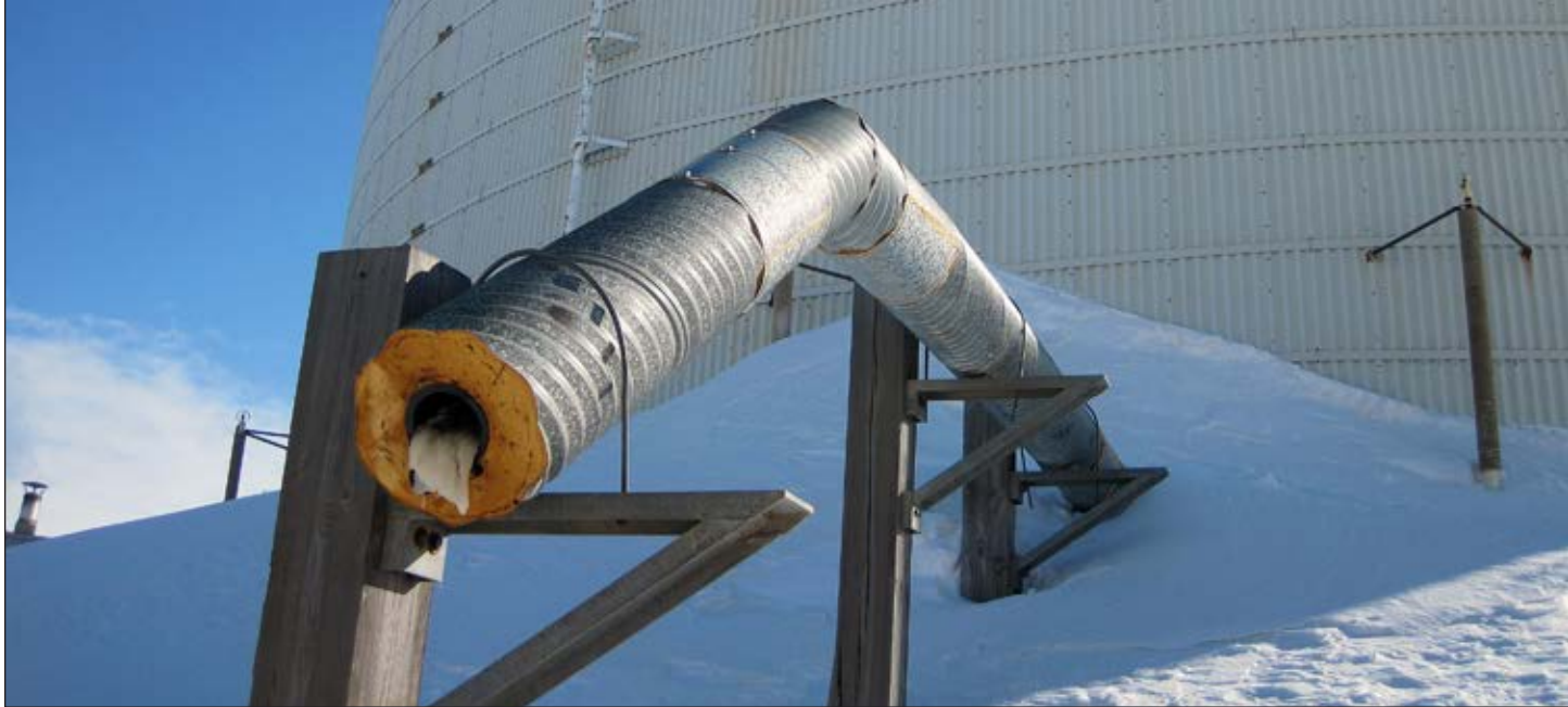
A water storage tank in Wainwright damaged by permafrost thaw. Jake Bell, 2014.
