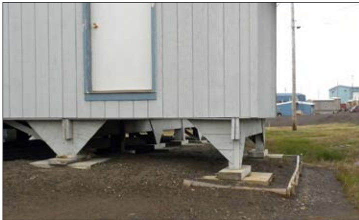
Frequent leveling of foundations is necessary. Mike Brubaker, 2013.
