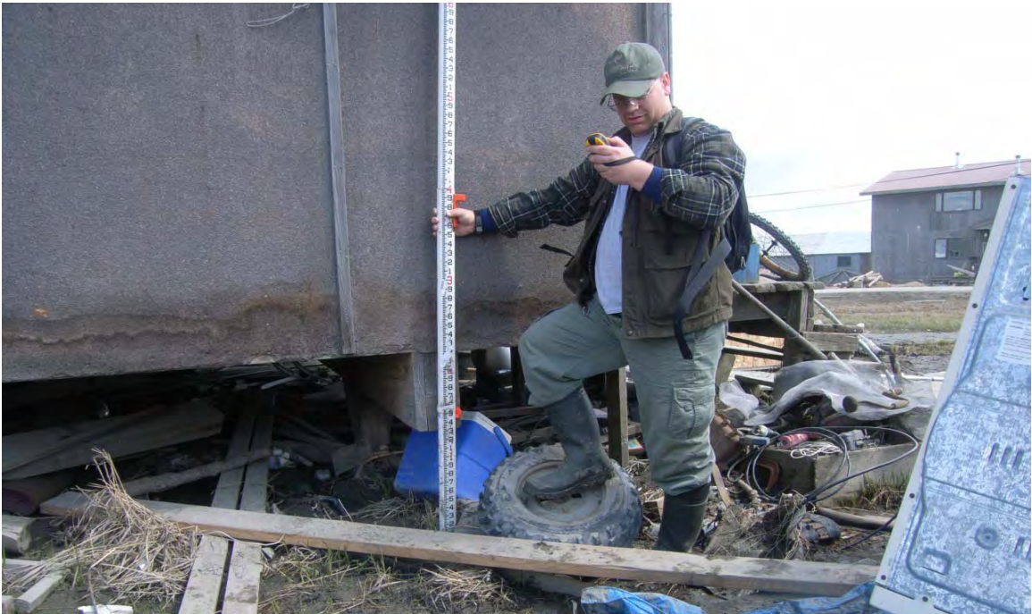
Figure 8: Water stain on wood siding, Emmonak, Poor, 2009
