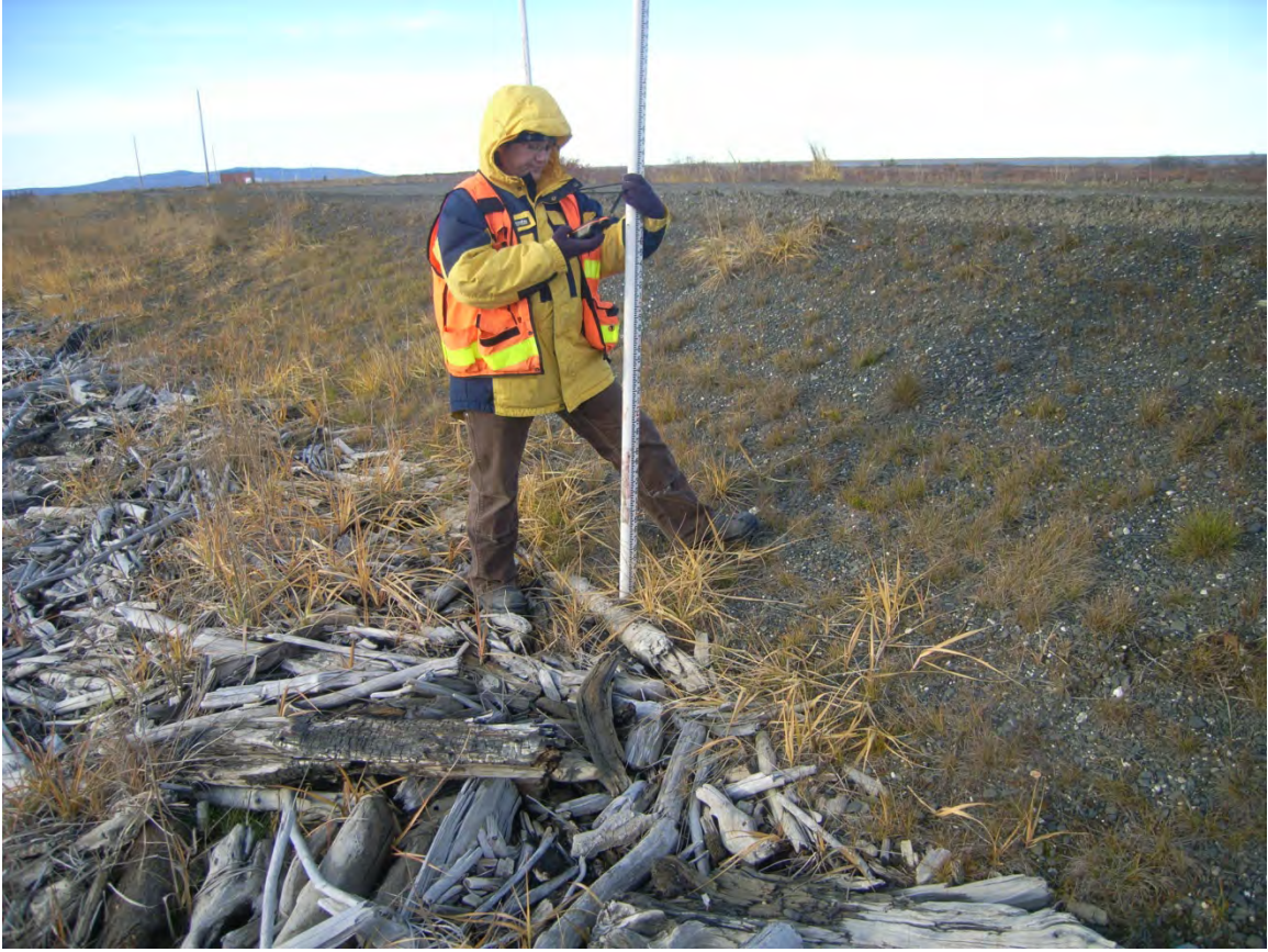
Figure 7: Debris line on road embankment, Poor, Shaktoolik, 2009.
