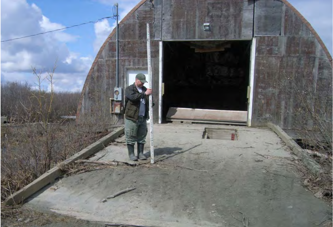
Figure 9: Debris line on access ramp, Fair. Emmonak, 2009.
